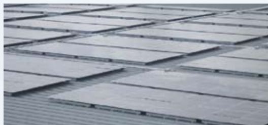
Thin-film PV cell panel installed at the new plant
